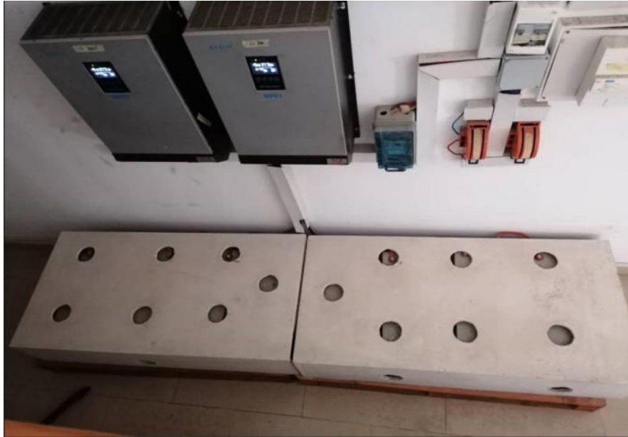
Figure 6. SOAC current UPS system
